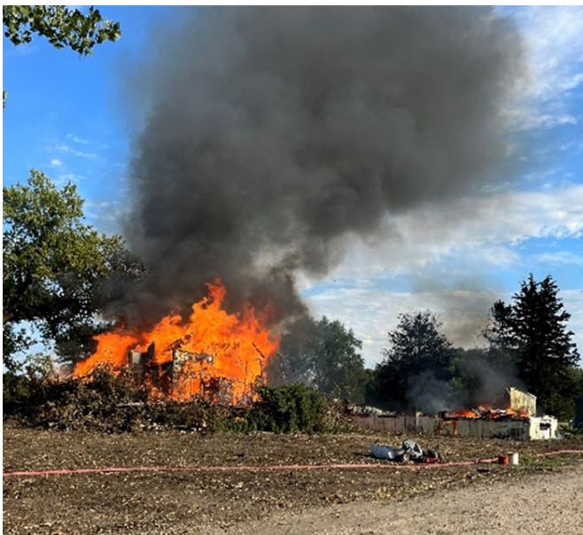
The City of Osmond acquisition project conducts a controlled burn demolition of properties acquired through the project.
