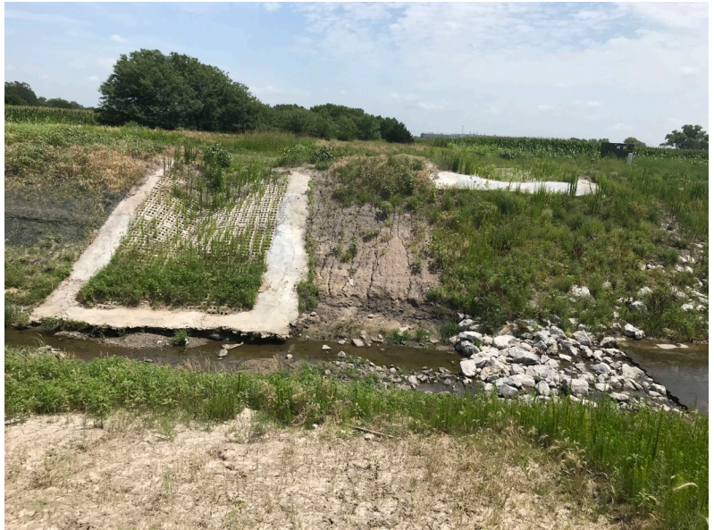
A bank stabilization project on Salt Creek near 56th and Morton streets in Lincoln was funded through the Hazard Mitigation Grant Program as a result of DR-4013, which was declared as result of the 2011 floods.
