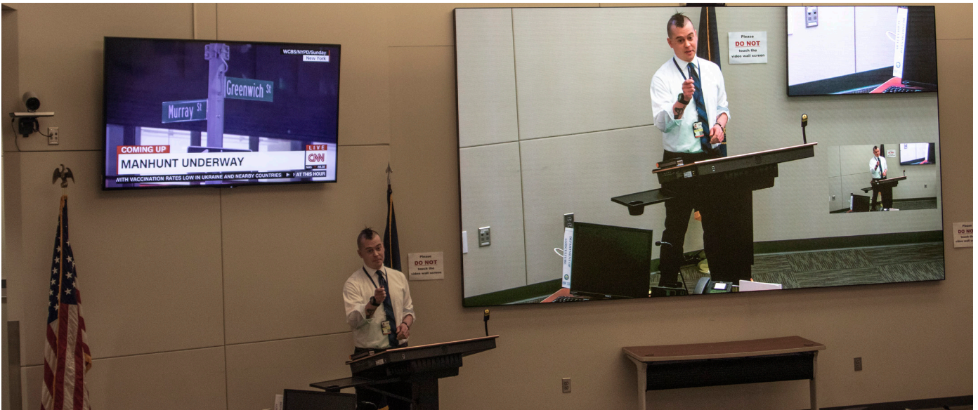
Many additions were made to the Nebraska Emergency Management Agency. Audio visual integrations and connections were established between the State Emergency Operations Center (SEOC) and conference rooms. Cameras were installed for video conferencing that enable staff to view operational activities in any of the other meeting spaces. A new podium was setup with laptop and presentation capabilities as well as a sound system that allows each emergency support function coordinator to brief during events or disasters, and to be heard in all other operational rooms as well as on webinars.
